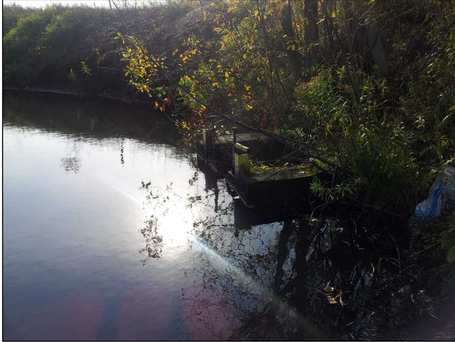
Photo 1: EDG Slag Pond inlet of hydraulic structure. Hydraulic structure consist of v-notch overflow weir that discharges into a 48-inch diameter corrugated metal pipe.
