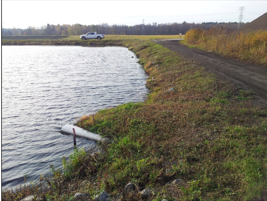
Photo 3: EDG South A-Pond inlet of hydraulic structure. Hydraulic structure consist of 18-inch diameter corrugated plastic pipe. Water flows through the hydraulic structure and discharges into a concrete sluice box prior to flowing through a Parshall flume structure.
