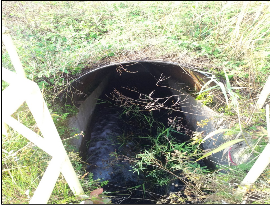
Photo 5: Water from the EDG South A-Pond flows into a 48-inch diameter corrugated metal pipe and combines with the flow from the EDG Slag Pond. The combined flows discharge into the EDG B-Pond.
