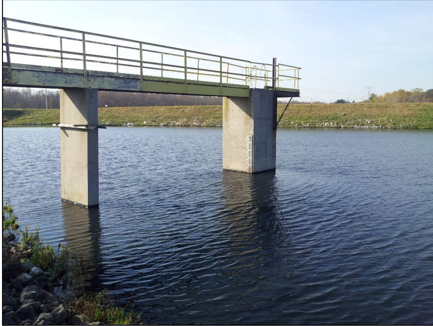
Photo 7: Water within the EDG B-Pond flows through an overflow weir structure. The water gravity flows through a 24-inch diameter corrugated metal pipe which discharges into the EDG C-Pond.
