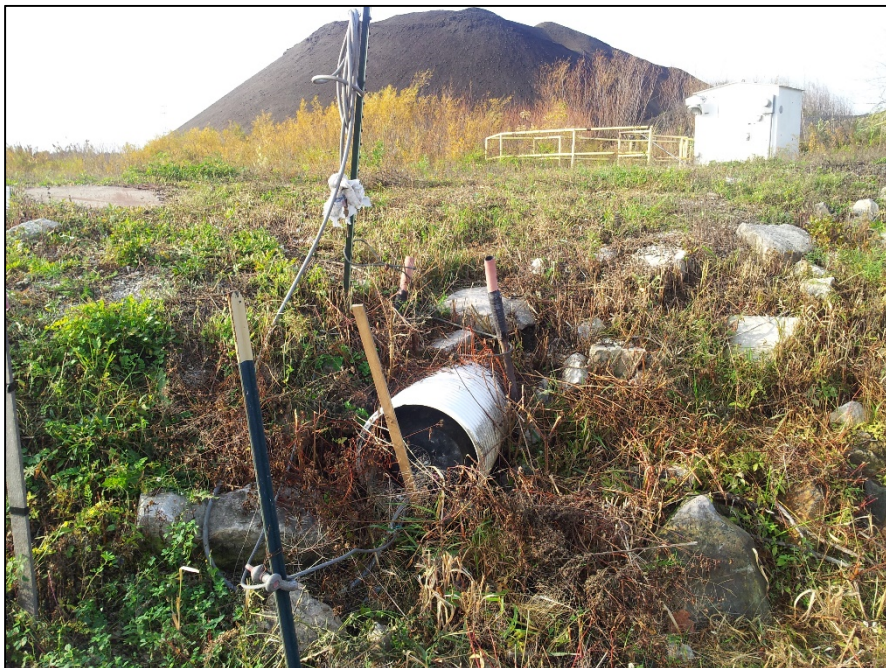
Photo 2: EDG North A-Pond inlet of hydraulic structure. Hydraulic structure consist of 18-inch diameter corrugated plastic pipe. The hydraulic structure is currently plugged.
