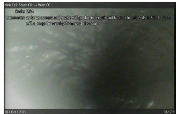
Survey Abandoned at 502.7 ft | as far as camera and nozzle will go due to length and friction from bends in
