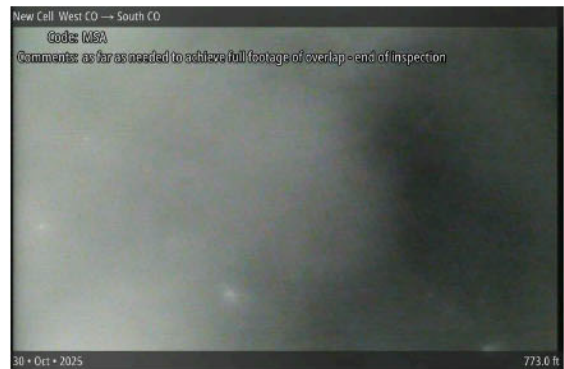
Survey Abandoned at 773.0 ft | as far as needed to achieve full footage of overlap - end of inspection
