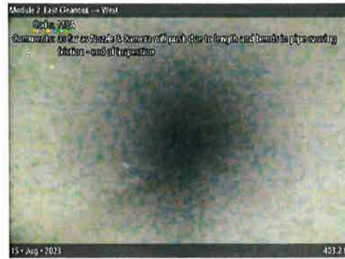
MSA at 403.2 ft | as far as Nozzle & Camera will push due to length and bends in pipe
