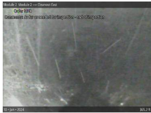
MSA at 365.2 ft | As far as needed for inspection - end of inspection
