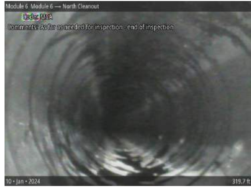
MSA at 319.7 ft | As far as camera will push - end of inspection
