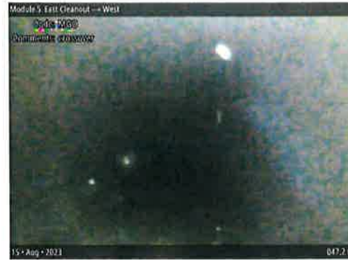
MGO at 044.2 ft | crossover
