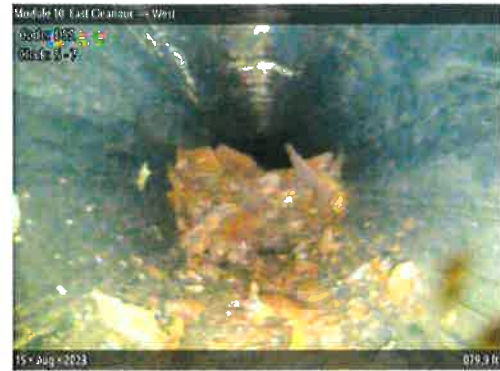
DSZ at 079.9 ft, 5 - 7 o'clock | Leachate Shale
