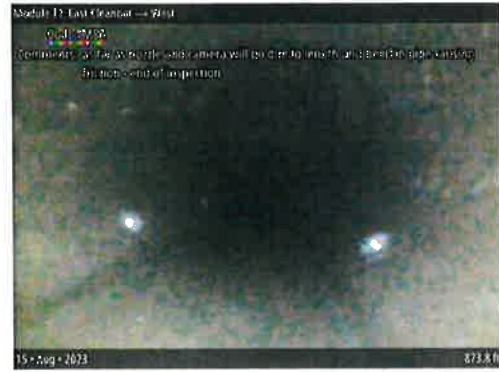
MSA at 873.8 ft | as far as nozzle and camera will go due to length and bend in pipe causing
