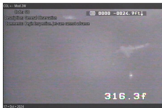
General Observation at 316.3 ft | Begin Inspection. Jet-cam cannot advance
