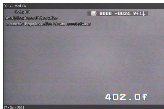
General Observation at 402.0 ft | Begin Inspection. Jet-cam cannot advance
