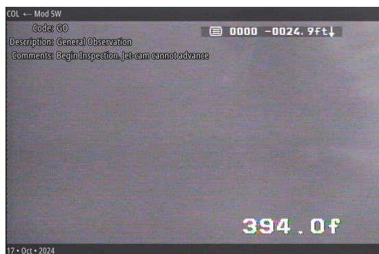
General Observation at 394.0 ft | Begin Inspection. Jet-cam cannot advance
