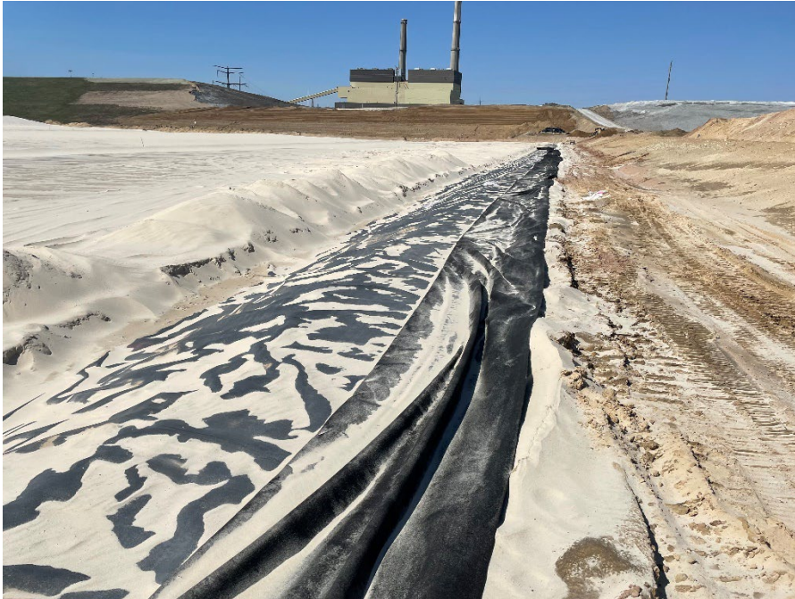
Photo 1: Plywood (2'x8'x0.5" sections wrapped in geotextile) placed at the northern edge of the existing geomembrane of Module 11 berm. (Looking west) (4/12/2023)
