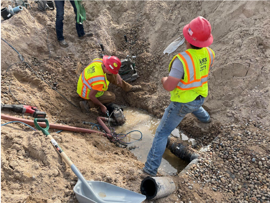
Photo 7: Removing an approximate 3-foot section of the leachate collection piping south of the “T” in Module 4. (Looking down) (4/28/2023)
