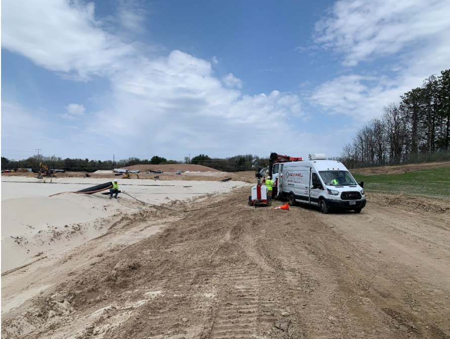
Photo 19: Jetting and televising the leachate collection pipes in Modules 10 and 11. (Looking north) (5/4/2023)
