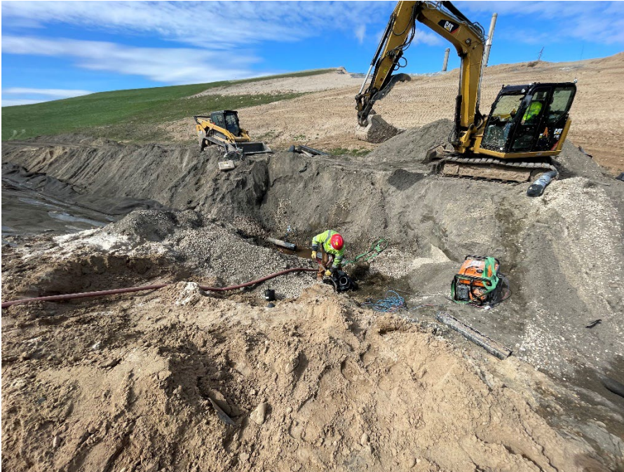
Photo 9: Removing an approximate 3-foot section of the leachate collection piping south of the Module 3 “T”. (Looking southwest) (5/2/2023)
