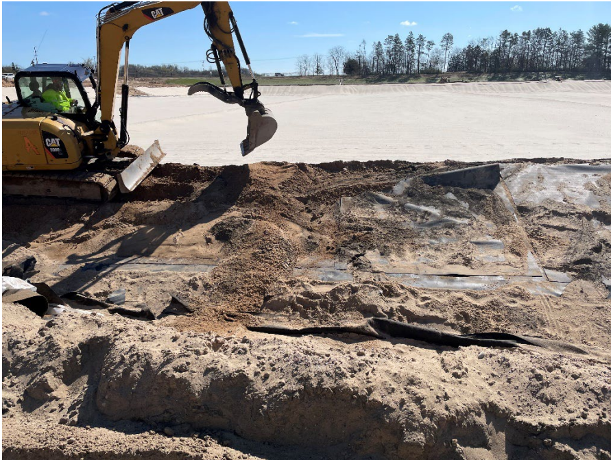
Photo 16: Removing the geomembrane flap on the berm between Modules 3/4 and 10/11. (Looking west) (5/3/2023)
