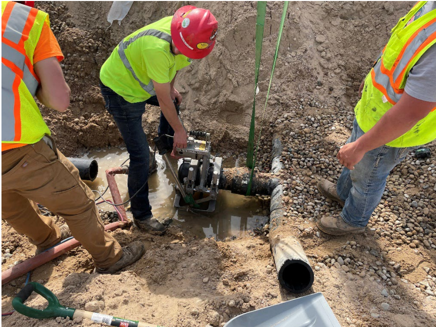
Photo 8: Fusion welding of the caps on the leachate collection pipe and cleanout in Module 4. (Looking west) (4/28/2023)
