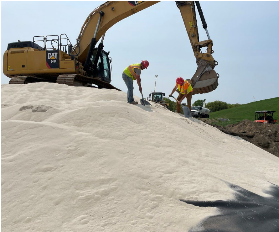
Photo 36: Drainage material placement on top of the geomembrane on the southwest temporary berm. (Looking southwest) (5/16/2023)
