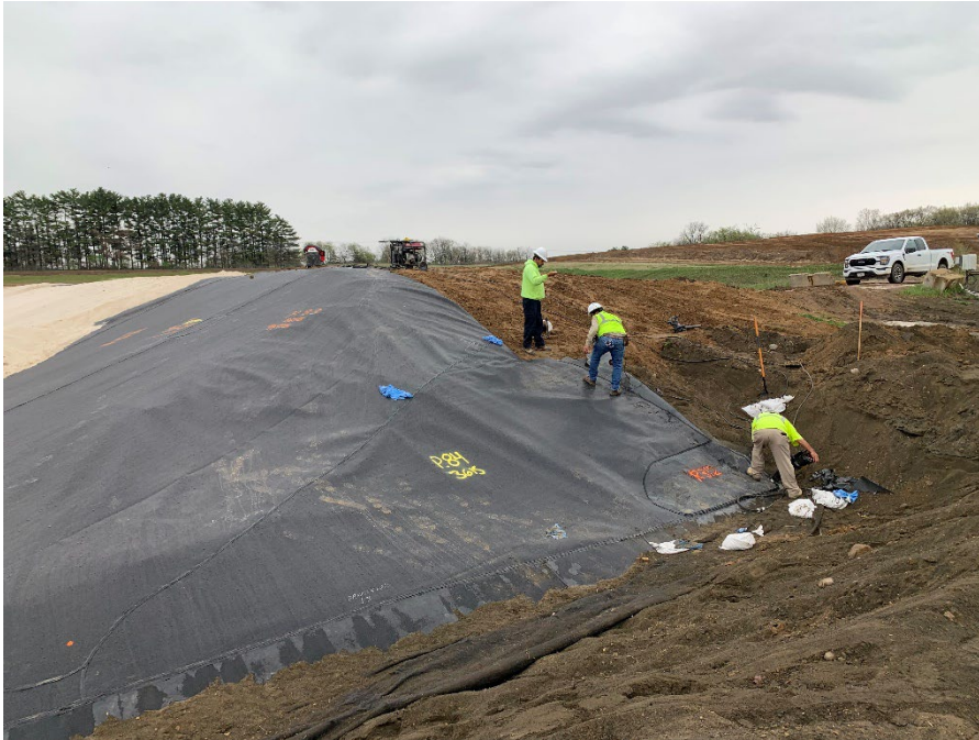
Photo 33: Southwest corner of Module 10 berm welded to existing flap of Module 2. (Looking southeast) (5/6/2023)
