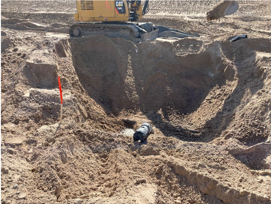
Photo 5: Removing and capping the leachate cleanout risers in Modules 3 and 4. (Looking west) (4/27/2023)
