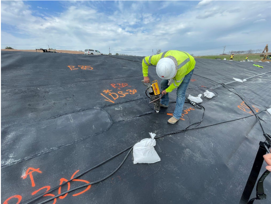
Photo 29: Extrusion welding of the geomembrane repairs on Module 11 north berm. (Looking northeast) (5/5/2023)
