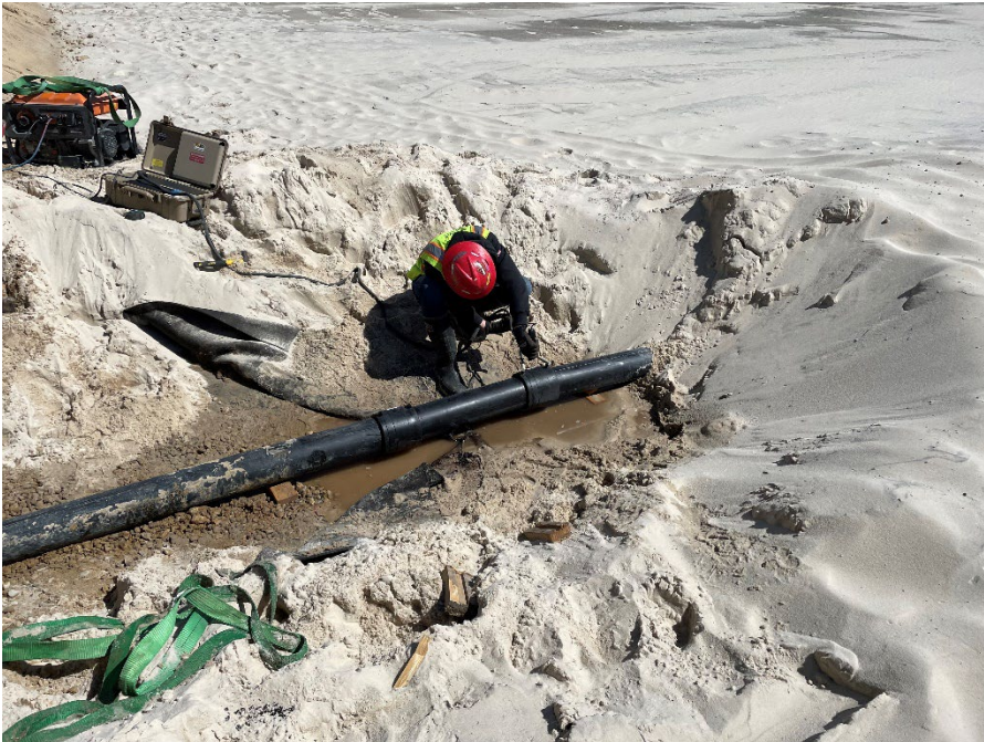
Photo 10: Fusion welding of the leachate collection pipe from Module 3 to Module 10. (Looking northeast) (5/2/2023)
