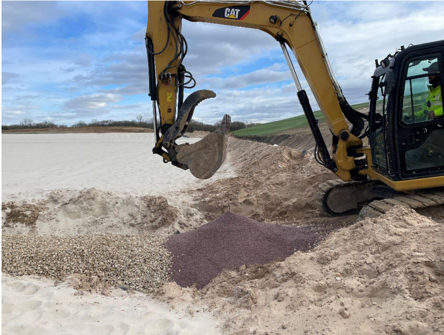
Photo 11: Placing layers of coarse aggregate bedding and filter material (1-foot-thick) on top of the leachate pipe connection in Module 11. (Looking south) (5/2/2023)
