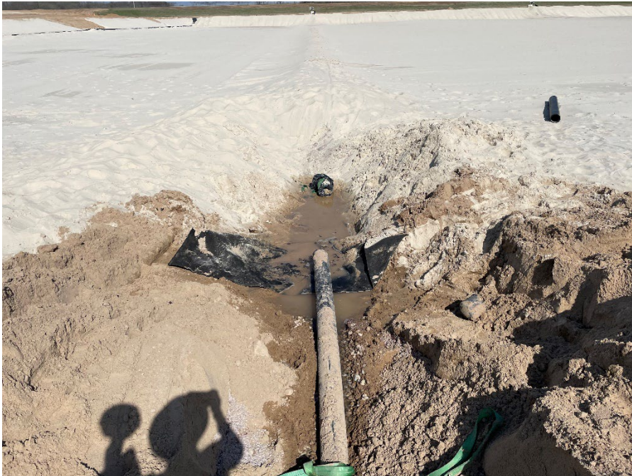
Photo 4: Exposing the east-west leachate collection pipes in preparation for pipe connections. (Looking east) (4/27/2023)
