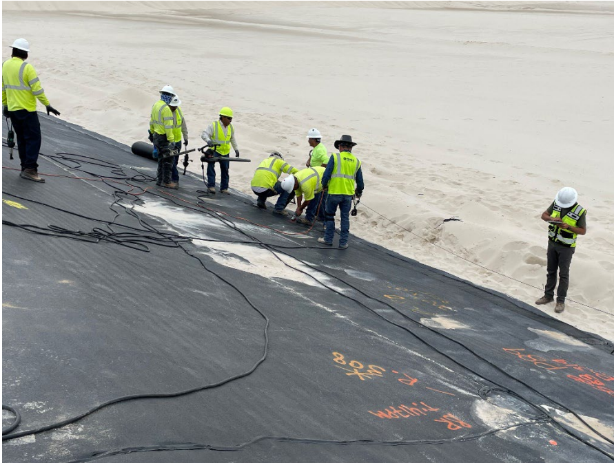
Photo 35: Collecting an additional destruct and performing repairs and vacuum box testing. (Looking southeast) (5/12/2023)
