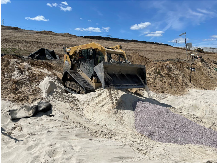
Photo 15: Placing layers of filter and drainage layer material (1-foot-thick) on top of the leachate pipe connection in Module 10. (Looking northwest) (5/3/2023)
