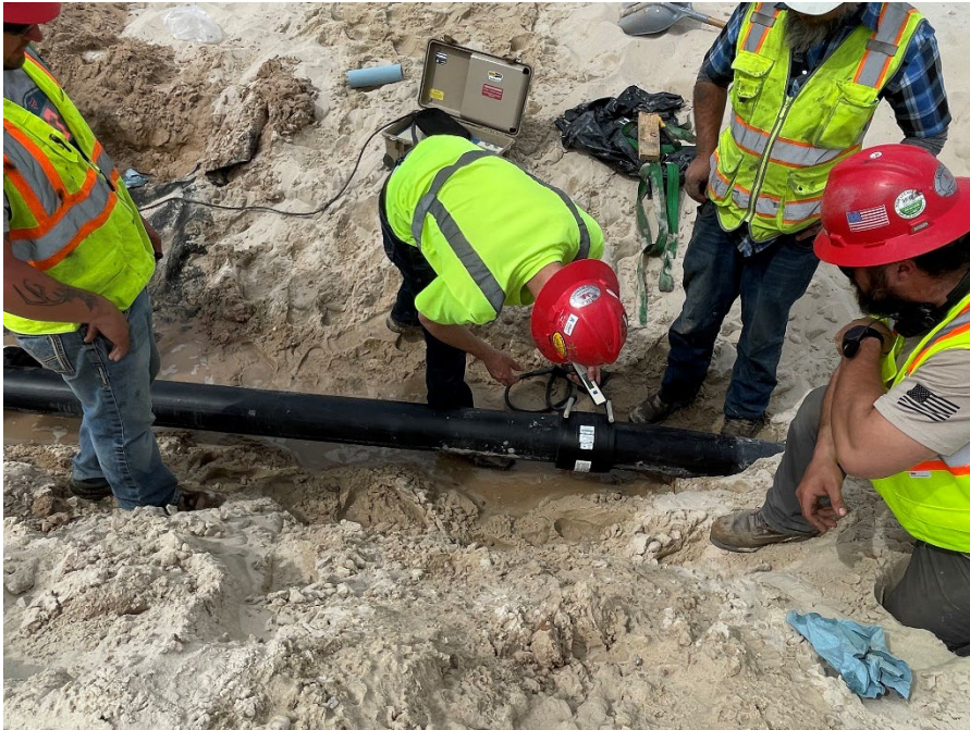
Photo 6: Electrofusion welding of east-west leachate collection pipe from Module 4 to Module 11. (Looking down) (4/28/2023)
