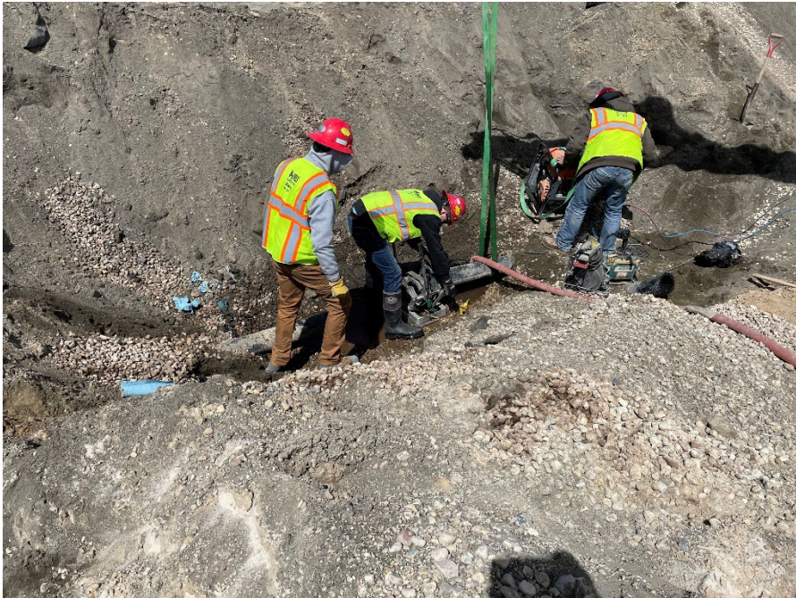
Photo 12: Fusion welding the caps on the leachate collection pipes and cleanout risers in Module 3 at leachate header plug location. (Looking northwest) (5/2/2023).
