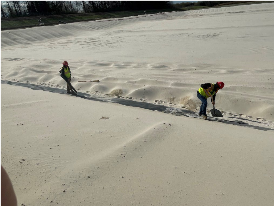
Photo 18: Cleaning surface of geomembrane at the north berm in preparation for the temporary geomembrane flap installation. (Looking southeast) (5/4/2023)
