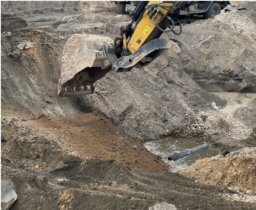
Photo 14: Placement of bentonite mixed sand for the leachate header plug. (Looking northwest) (5/2/2023)
