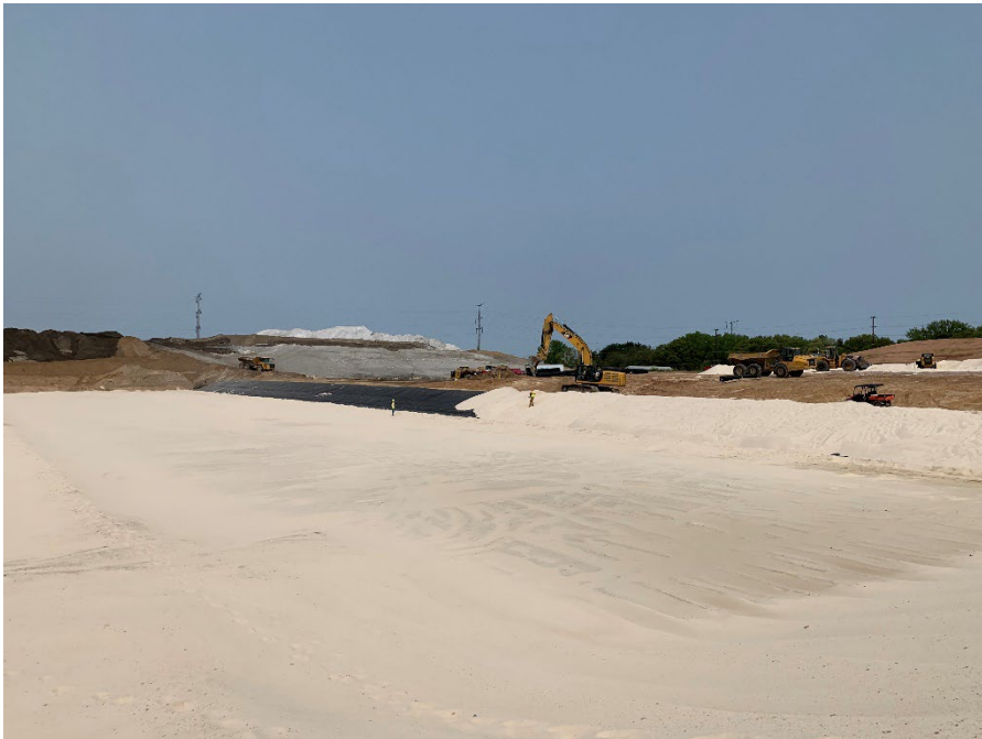
Photo 38: Drainage material placement on top of the geomembrane on the temporary north berm. (Looking northwest) (5/17/2023)
