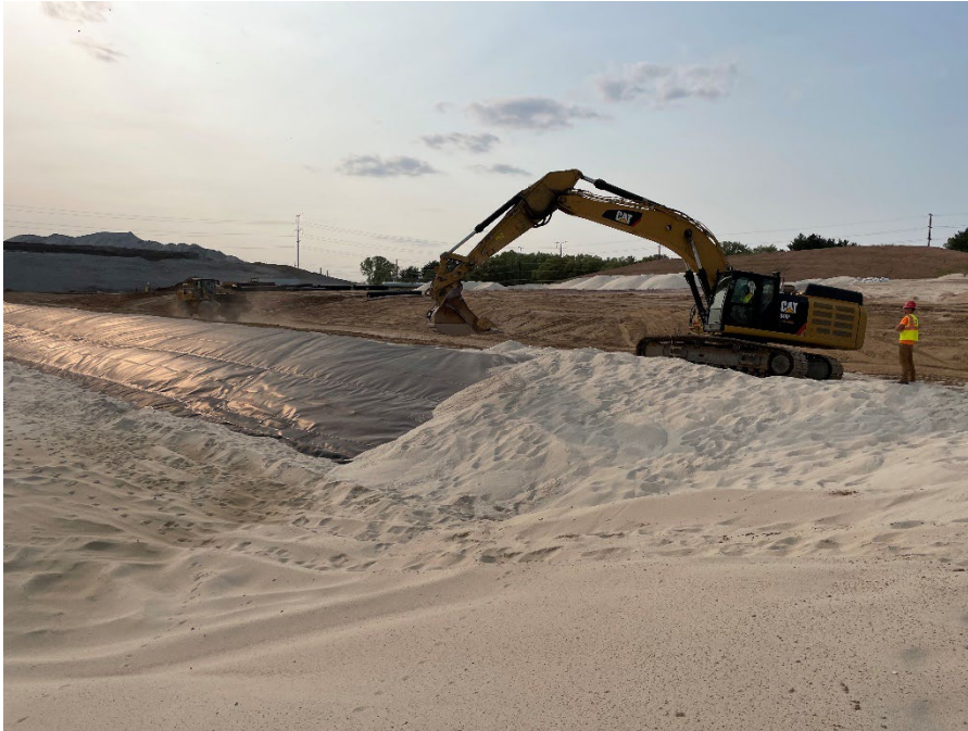
Photo 37: Drainage material placement on top of the geomembrane on the temporary north berm. (Looking northwest) (5/16/2023)
