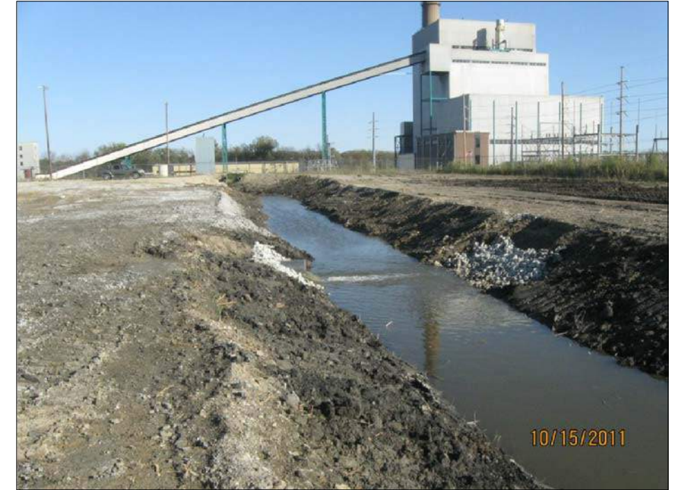
18-INCH HDPE POND DISCHARGE PIPE (OUTLET)
