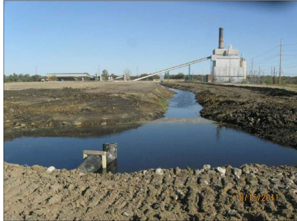
18-INCH HDPE CHANNEL DISCHARGE PIPE (INLET)
