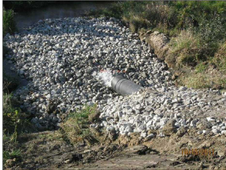
18-INCH HDPE CHANNEL DISCHARGE PIPE (OUTLET)
