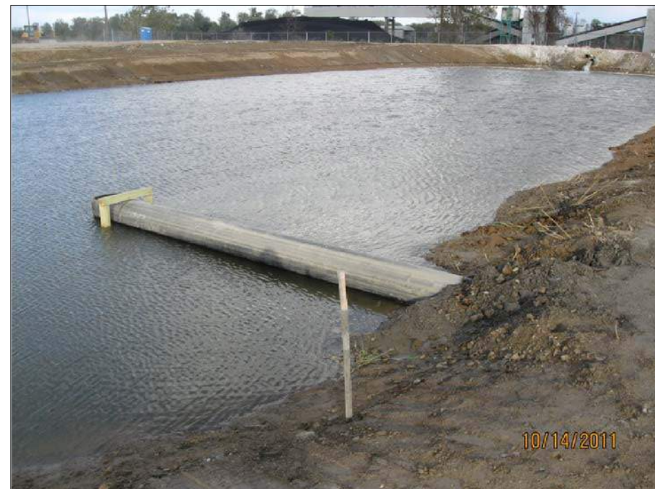
18-INCH HDPE POND DISCHARGE PIPE (POND SIDE)
