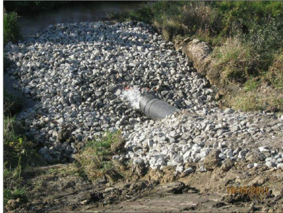
18-INCH HDPE CHANNEL DISCHARGE PIPE (OUTLET)
