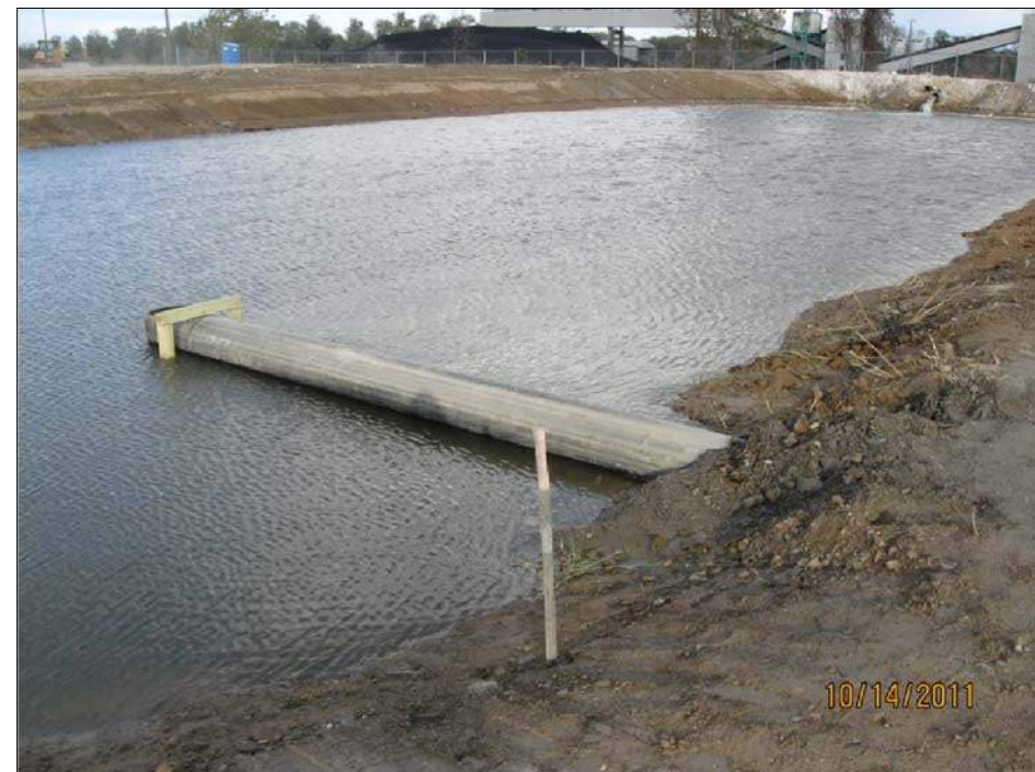
18-INCH HDPE POND DISCHARGE PIPE (POND SIDE)
