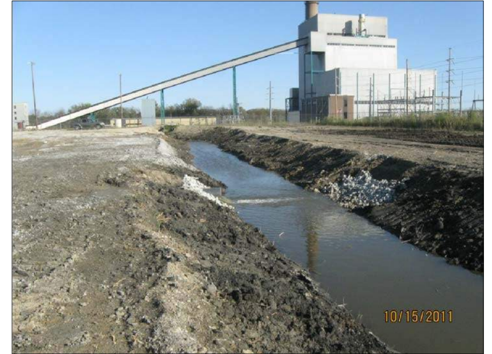
18-INCH HDPE POND DISCHARGE PIPE (OUTLET)
