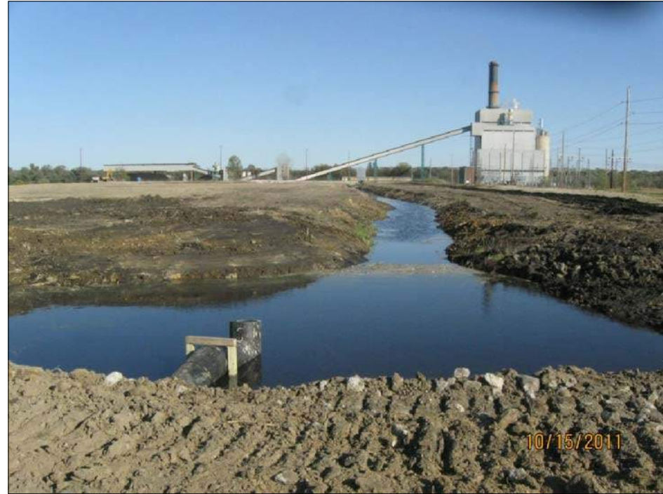
18-INCH HDPE CHANNEL DISCHARGE PIPE (INLET)
