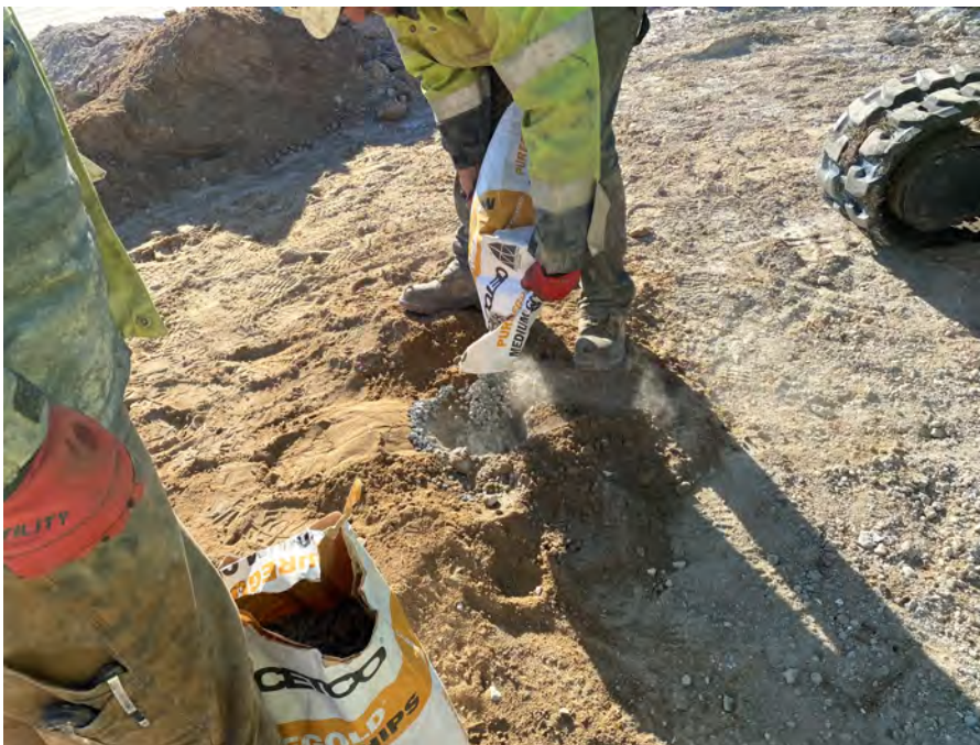
Photo 4: Completing abandonment of MW-313X. MW-313 was later installed 1.5 feet east of MW-313X.
